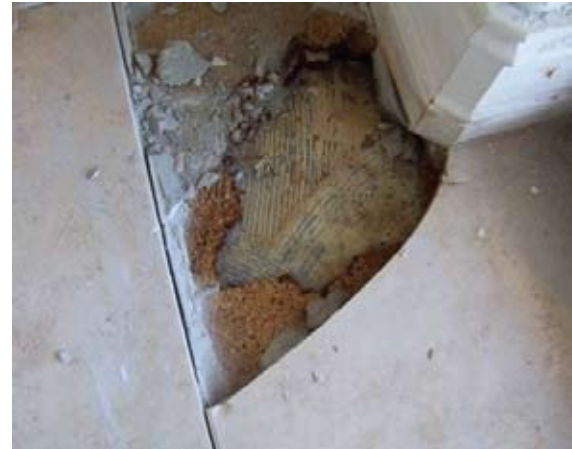
Above: The stained grout in this installation was removed following water seepage from a nearby window.
